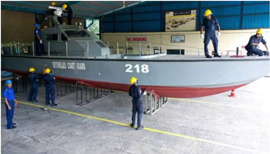
Construction of a IPC for Republic of Seychelles Coast Guard at NBBY
